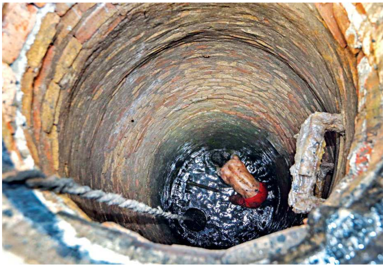
A worker of Dhaka Water Supply and Sewerage Authority (Wasa) cleaning a sewerage line in the capital to ensure uninterrupted drainage facilities to the city dwellers. He has no safety gear when even the inhalation of the fumes inside such manholes could become fatal. The photo was taken on the Holy Cross Road recently.
