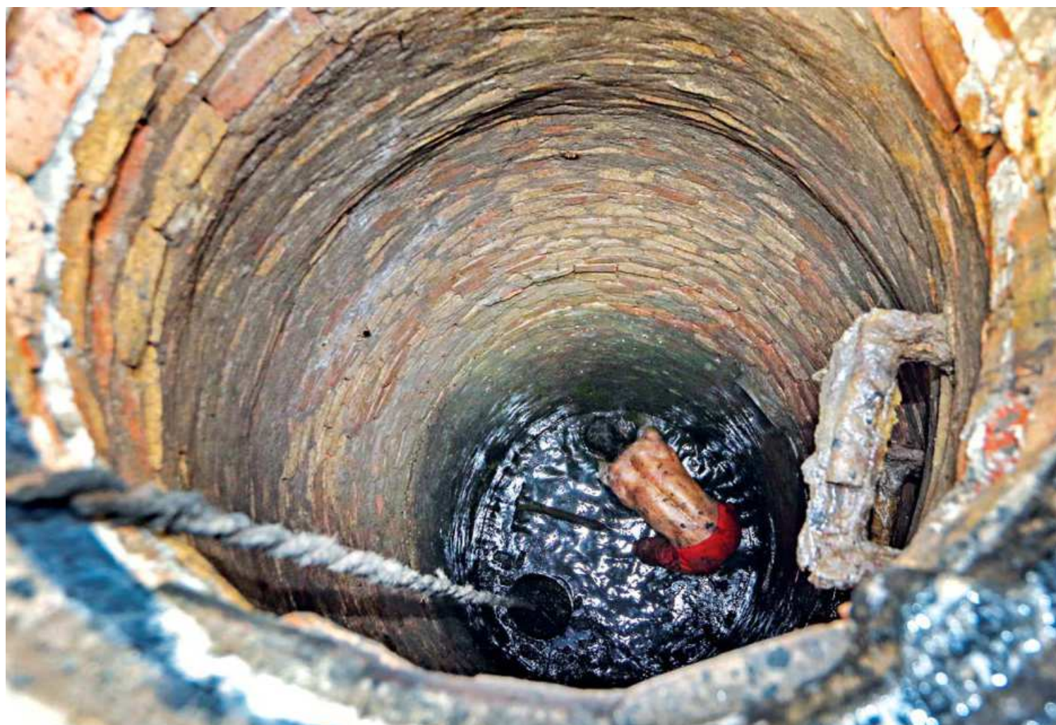
A worker of Dhaka Water Supply and Sewerage Authority (Wasa) cleaning a sewerage line in the capital to ensure uninterrupted drainage facilities to the city dwellers. He has no safety gear when even the inhalation of the fumes inside such manholes could become fatal. The photo was taken on the Holy Cross Road recently.
