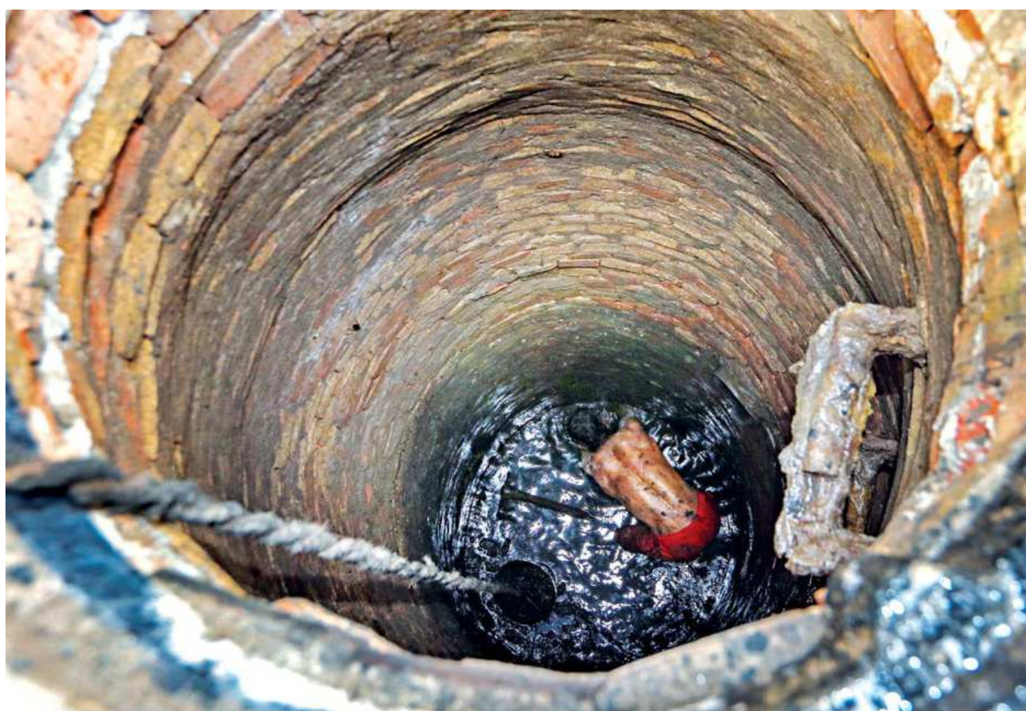
A worker of Dhaka Water Supply and Sewerage Authority (Wasa) cleaning a sewerage line in the capital to ensure uninterrupted drainage facilities to the city dwellers. He has no safety gears when even the inhalation of the fumes inside such manholes could become fatal. The photo was taken on the Holy Cross Road recently.
