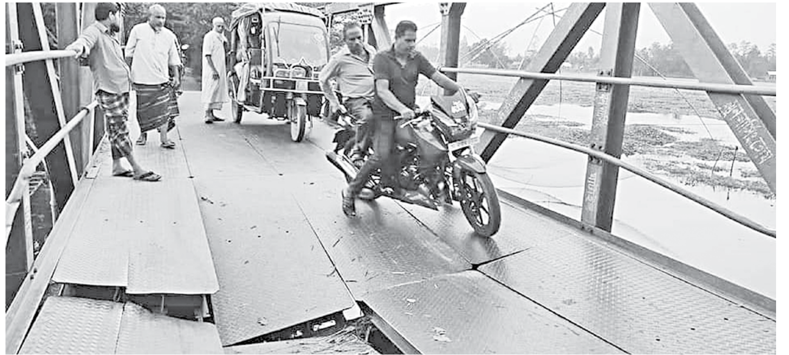
This recent photo shows pedestrians and vehicles cross the damaged portion of this bailey bridge on Kalihati-Dhalapara-Barachaona road in Tangail's Kalihati upazila amid risk of fatal accidents.
