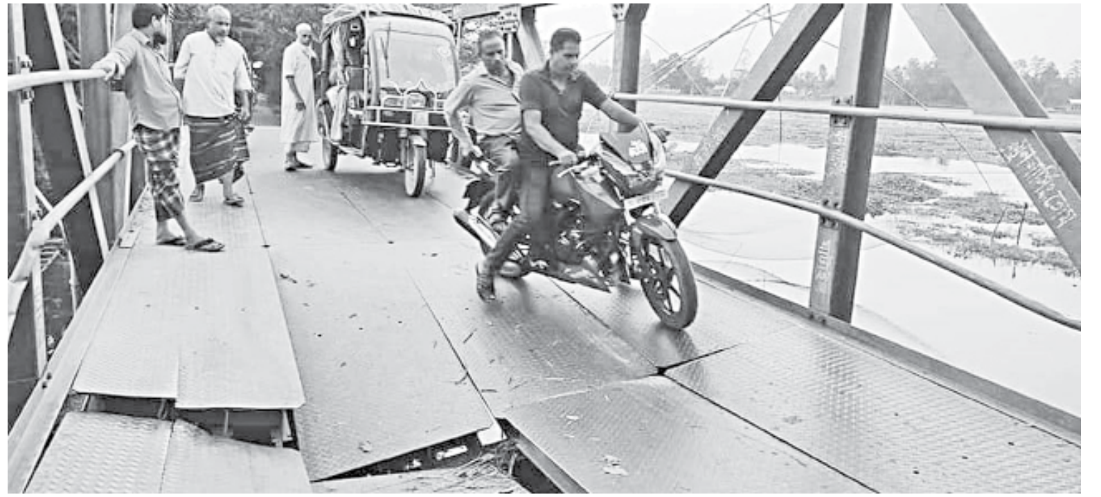
This recent photo shows pedestrians and vehicles cross the damaged portion of this bailey bridge on Kalihati-Dhalapara-Barachaona road in Tangail's Kalihati upazila amid risk of fatal accidents.
