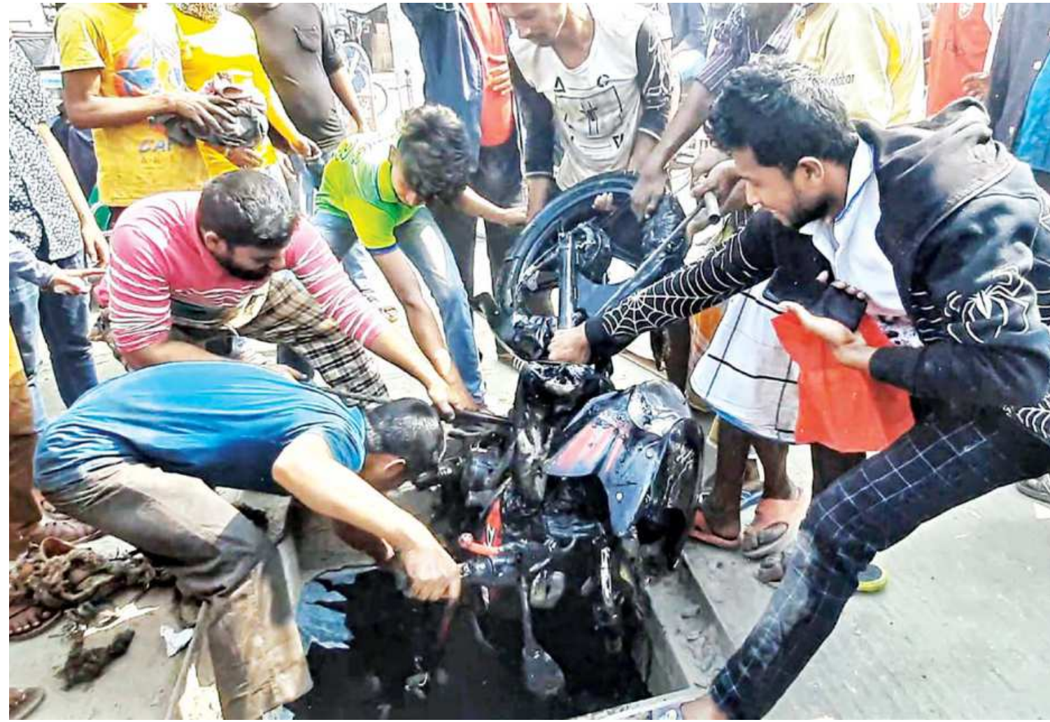
A motorcycle being pulled out of a manhole on KDA Avenue in Khulna city after a biker fell into it yesterday. The accident happened as the authorities concerned removed the cover for work in sewerage lines on both sides of the road.
