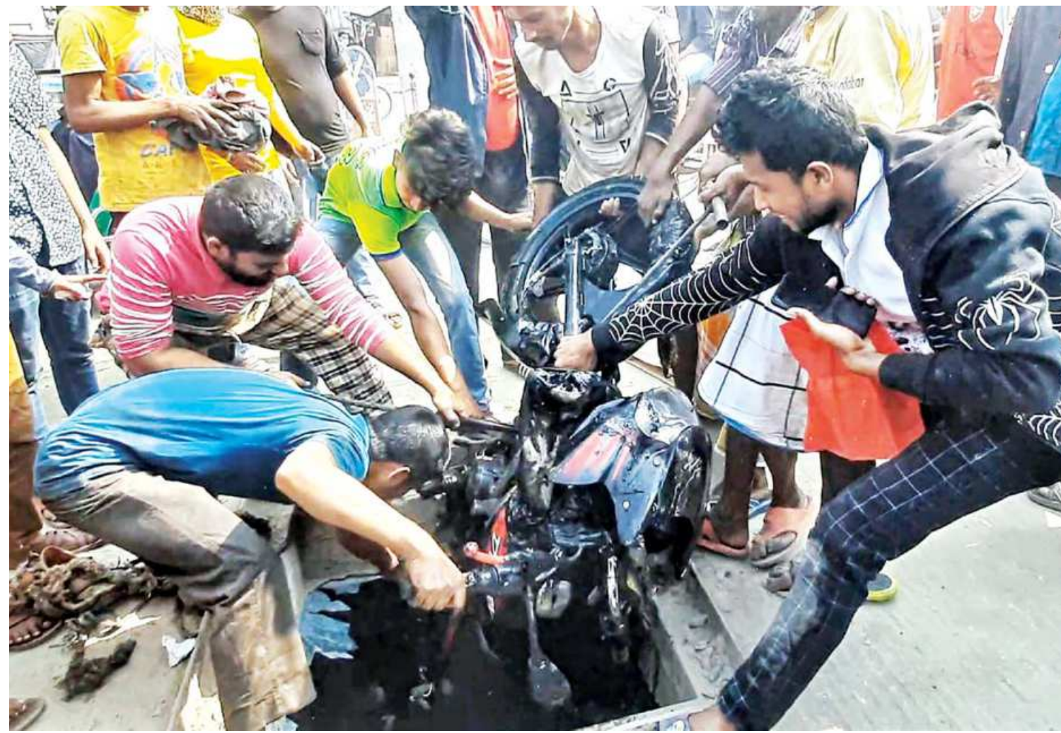
A motorcycle being pulled out from a manhole on KDA Avenue in Khulna city after a biker fell into it yesterday. The accident happened as the authorities concerned removed the cover for work in sewerage lines on both sides of the road.
