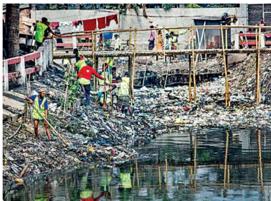
The workers of Dhaka North City Corporation cleaning Ramchandrapur canal in the capital's Adbor area yesterday. The corporation was recently entrusted with the task of maintaining the canal.
