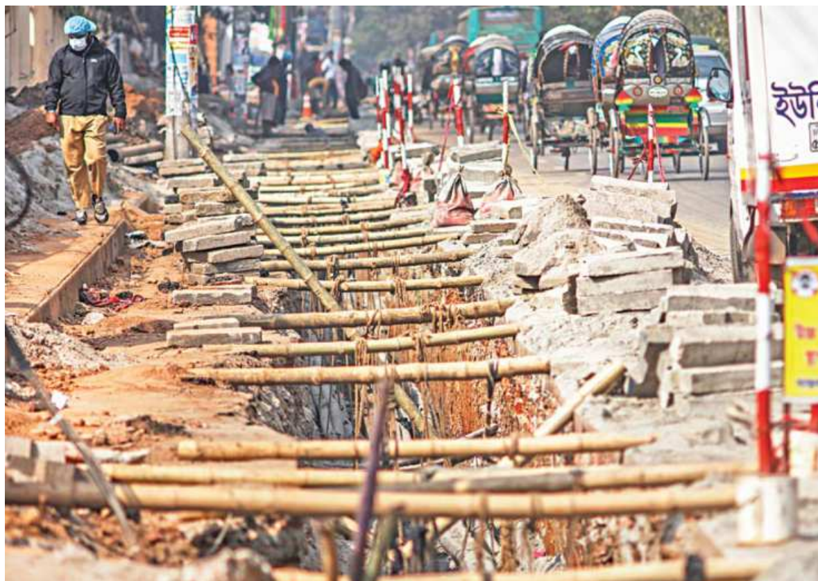
Just one wrong step and that passerby would fall into the hole dug for installing underground cables. This project by DPDC at Sat Masjid Road has been under the works for a month. With no proper barricades, pedestrians and vehicles are at risk when commuting through this road.
