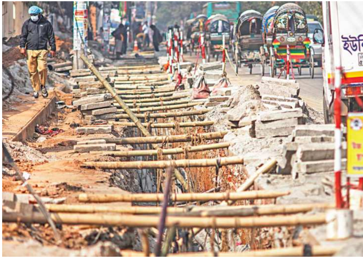
Just one wrong step and that passerby would fall into the hole dug for installing underground cables. This project by DPDC at Sat Masjid Road has been under the works for a month. With no proper barricades, pedestrians and vehicles are at risk when commuting through this road.
