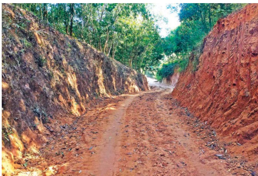
In the name of repairing Pachpir Jhali Road, 2.09 lakh cubic feet of hills were cut using government funds by a local union parishad member in Moulvibazar. Finding out, the DoE yesterday fined him Tk 13.12 lakh.
