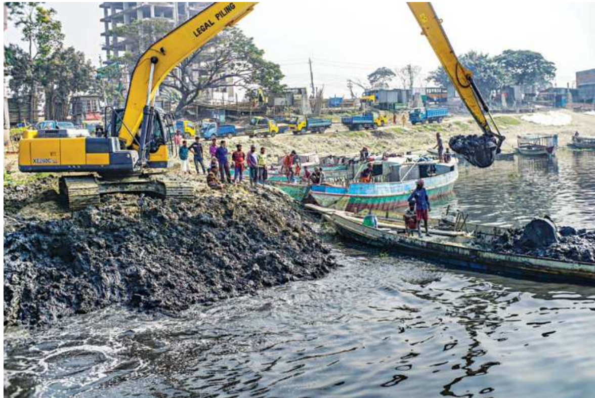
Workers of the BIWTA excavating sediment to increase the navigability of the Turag river in and around its Mirpur's Diabari landing station yesterday. The soil is later sold.
