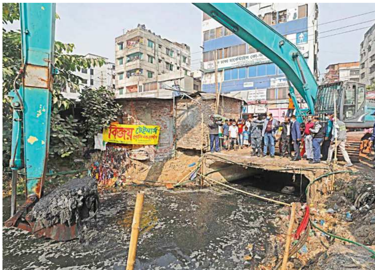
DNCC Mayor Atiqul Islam firsthand observed yesterday's drive to recover Ibrahimpur canal from encroachers. He said all illegal structures will be demolished to save the waterways, and authorities will conduct such drives for other canals as well.
