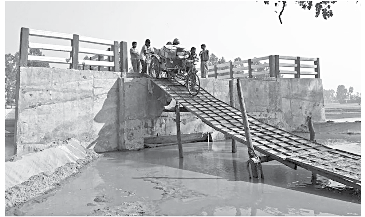
Due to lack of approach roads on both sides of the bridge over the Jinjiram river in Kurigram's Roumari upazila, people face untold sufferings.
