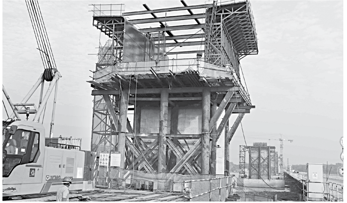
An under-construction pier of the Eighth Bangladesh-China Friendship Bridge, which was previously set to be open this month, over the Kacha river in Pirojpur. According to a newly set deadline, the Tk 822-crore bridge might get completed by June next year. The photo was taken recently.
