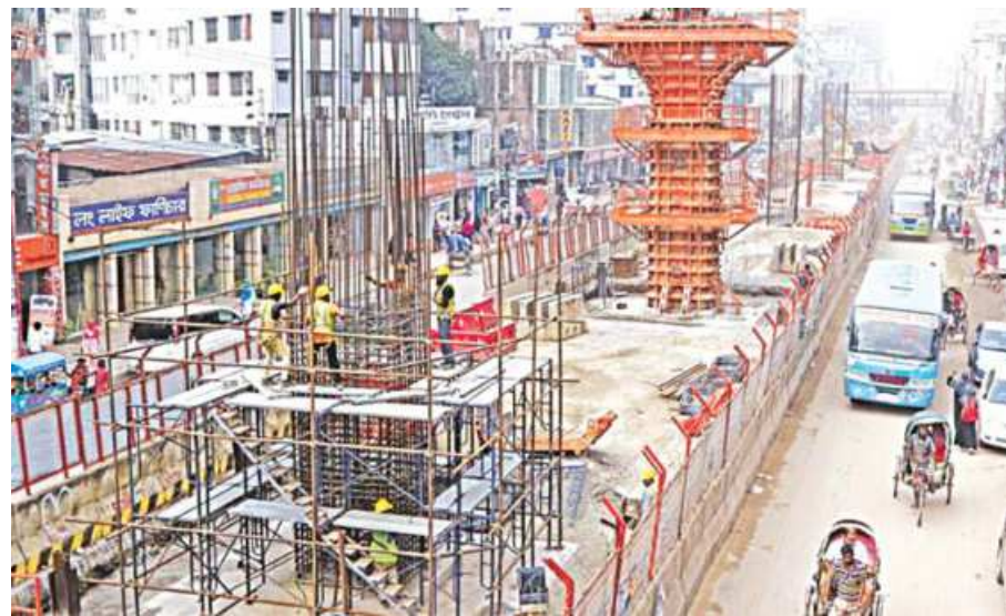
File photo of a construction site of the Dhaka Metro Rail project.
