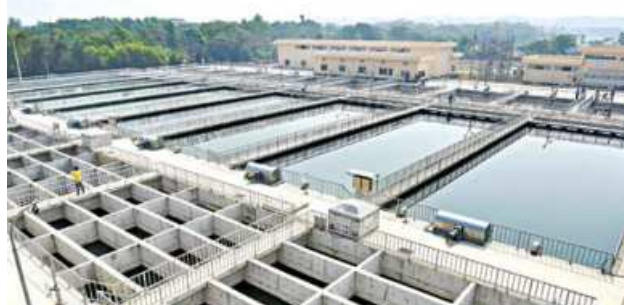
Modunaghat Water Treatment plant is currently withdrawing nine crore litres of water a day from the Halda river.
