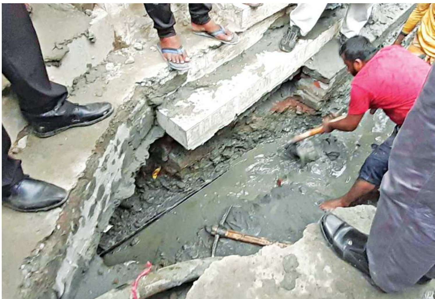
Workers hired by Titas Gas company dig out a gas pipeline at the main entrance to Pashchim Talla Baitus Salam Mosque in Narayanganj yesterday. The company is carrying out the digging work as part of its investigation into the Friday's fire incident that led to the deaths of 28 people.
