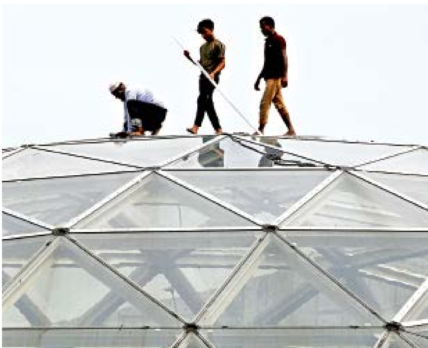
Standing atop a dome-shaped structure, these three workers go about their daily grind on a Sunday morning in Bijoy Sarani. Like them, thousands in the capital work in the construction sector without any safety measures and equipment, putting their lives at risk.
