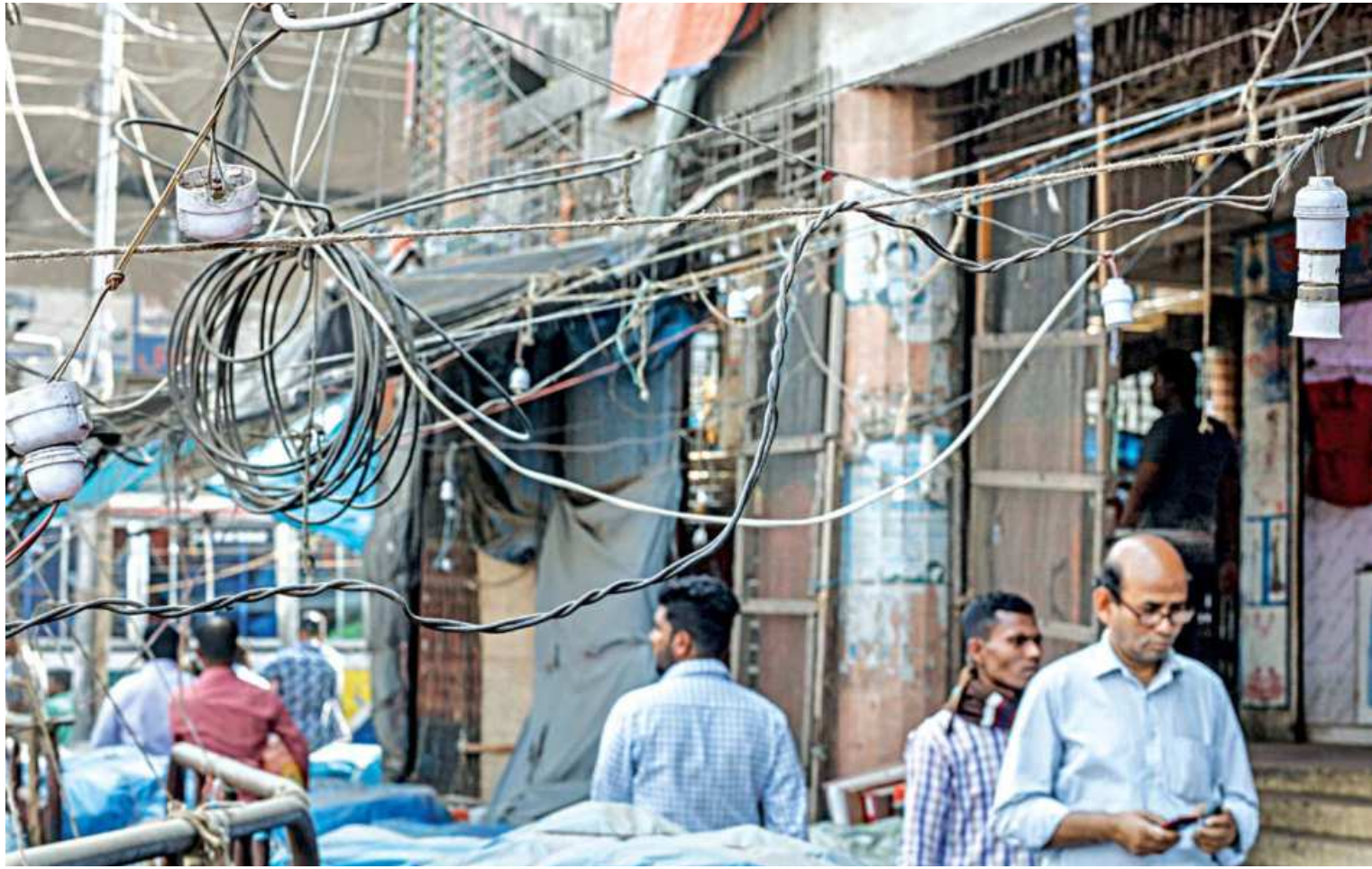
WIRES HAYWIRE... The ubiquity of cables and wires hanging above Dhaka streets have desensitised residents of the danger they possess, not to mention the sheer eyesore. In this photo taken from Gulistan yesterday, loose cables and unprotected light holders can be seen dangling above footpaths. How they got there is another story of irregularity -- they were put up by a "syndicate" that illegally occupies the pavement and rents it out to streetside vendors. PHOTO: RASHED SHUMON
