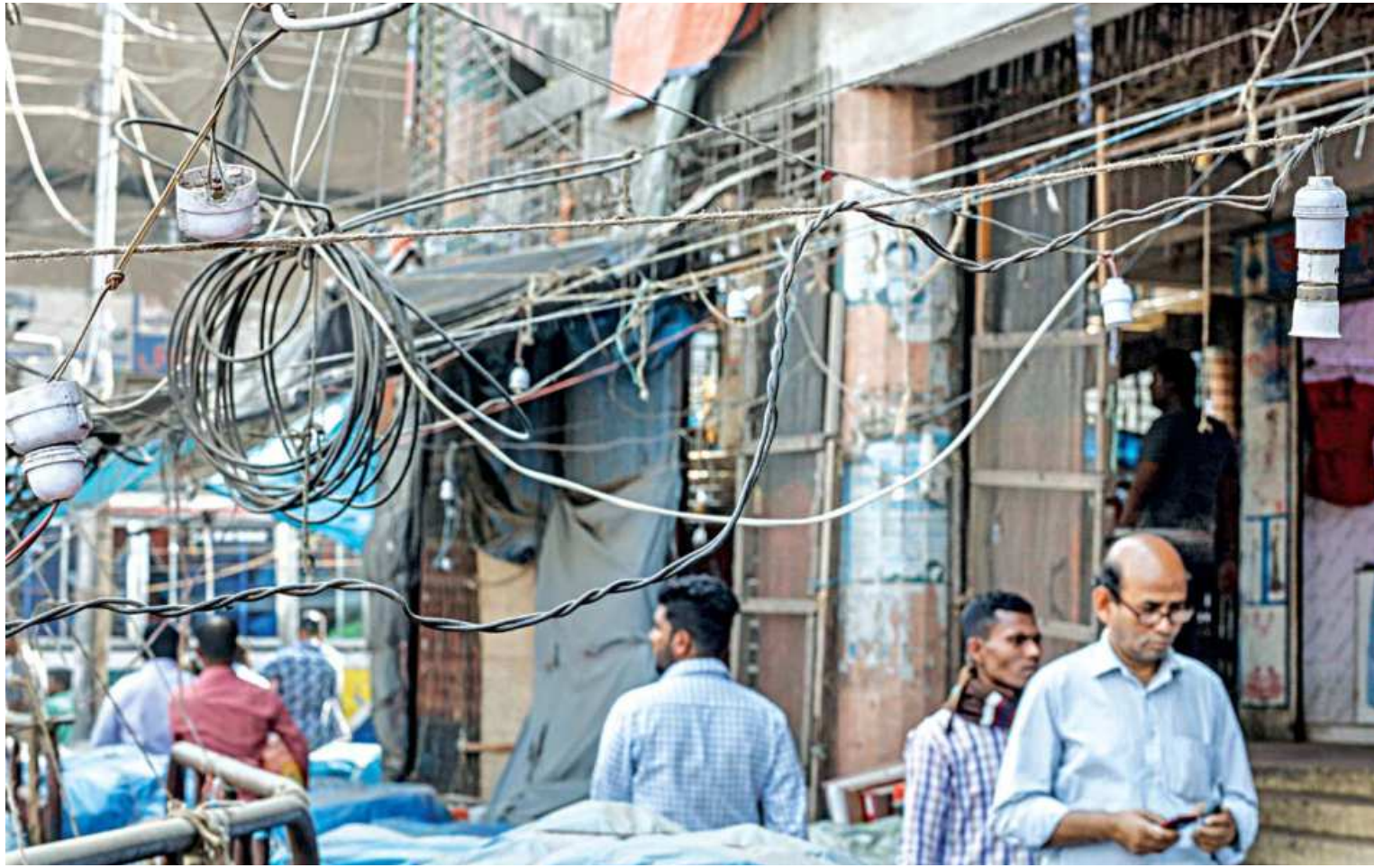
WIRES HAYWIRE... The ubiquity of cables and wires hanging above Dhaka streets have desensitised residents of the danger they possess, not to mention the sheer eyesore. In this photo taken from Gulistan yesterday, loose cables and unprotected light holders can be seen dangling above footpaths. How they got there is another story of irregularity -- they were put up by a "syndicate" that illegally occupies the pavement and rents it out to streetside vendors. PHOTO: RASHED SHUMON
