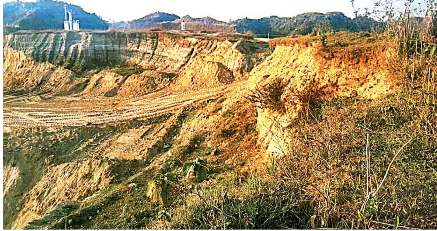
Part of a hill being flattened in Jongol Salimpur area of Chattogram's Sitakunda. The Chattogram Development Authority has continued cutting the hill although the Department of Environment imposed a fine of Tk 10 crore on it in January. The photo was taken recently.
