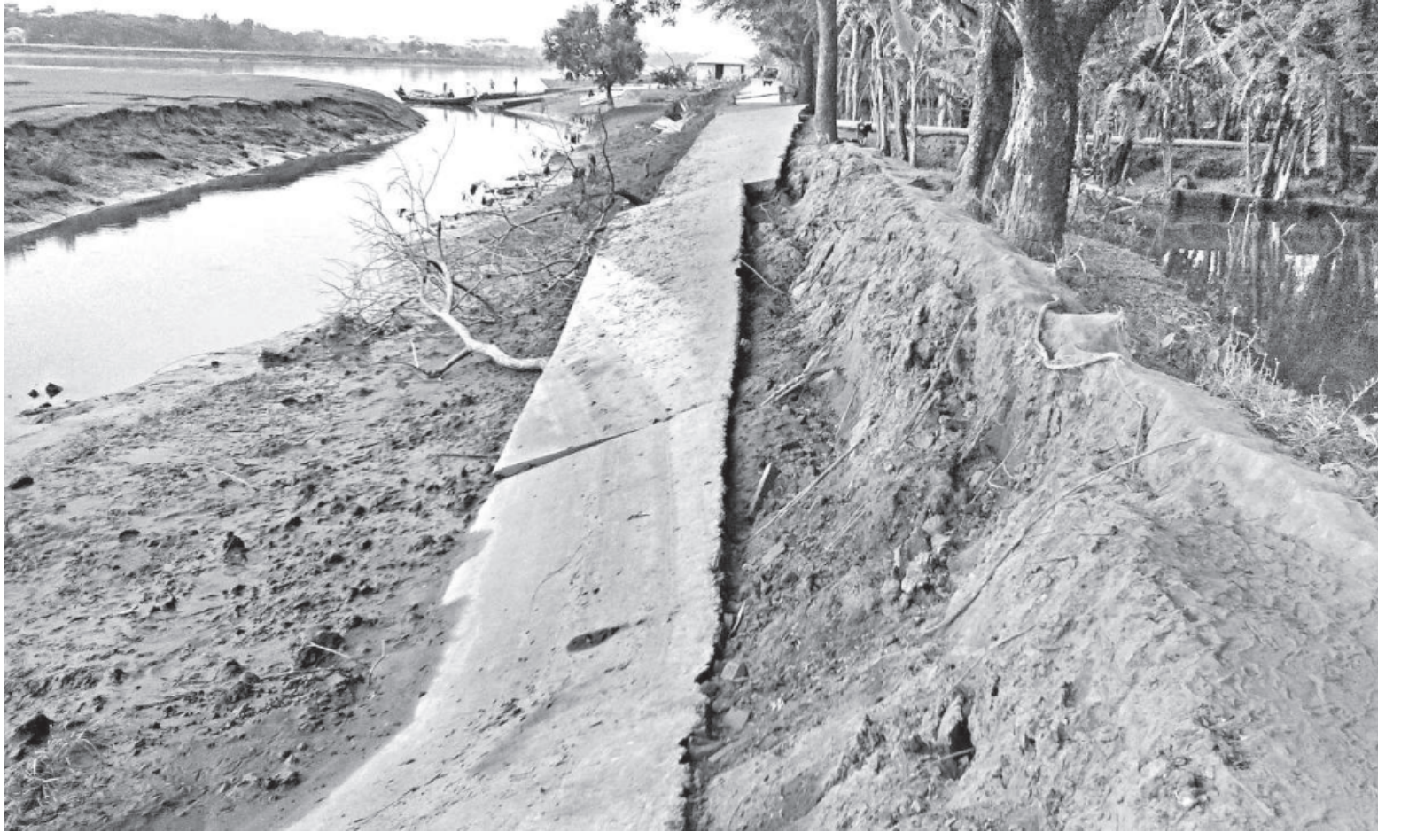
A collapsed portion of the road at Tegachia Kheyaghat on the Sonatala river in Patuakhali's Kalapara upazila.
