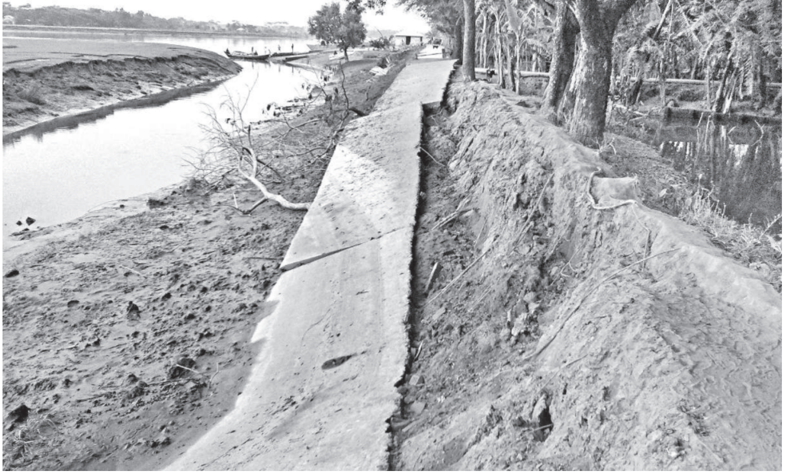
A collapsed portion of the road at Tegachia Kheyaghat on the Sonatala river in Patuakhali's Kalapara upazila.
