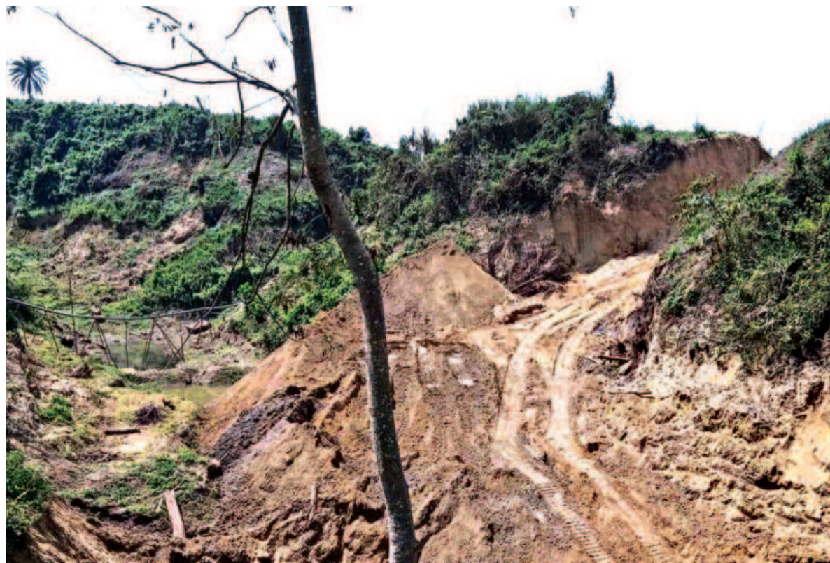
Hills being razed in Barabkunda of Chattogram's Sitakunda upazila. Despite a crackdown and fines on various businesses for hill-cutting over the past three years, hills continue to be razed in Mirsarai and Sitakunda upazilas. The photo was taken recently.
