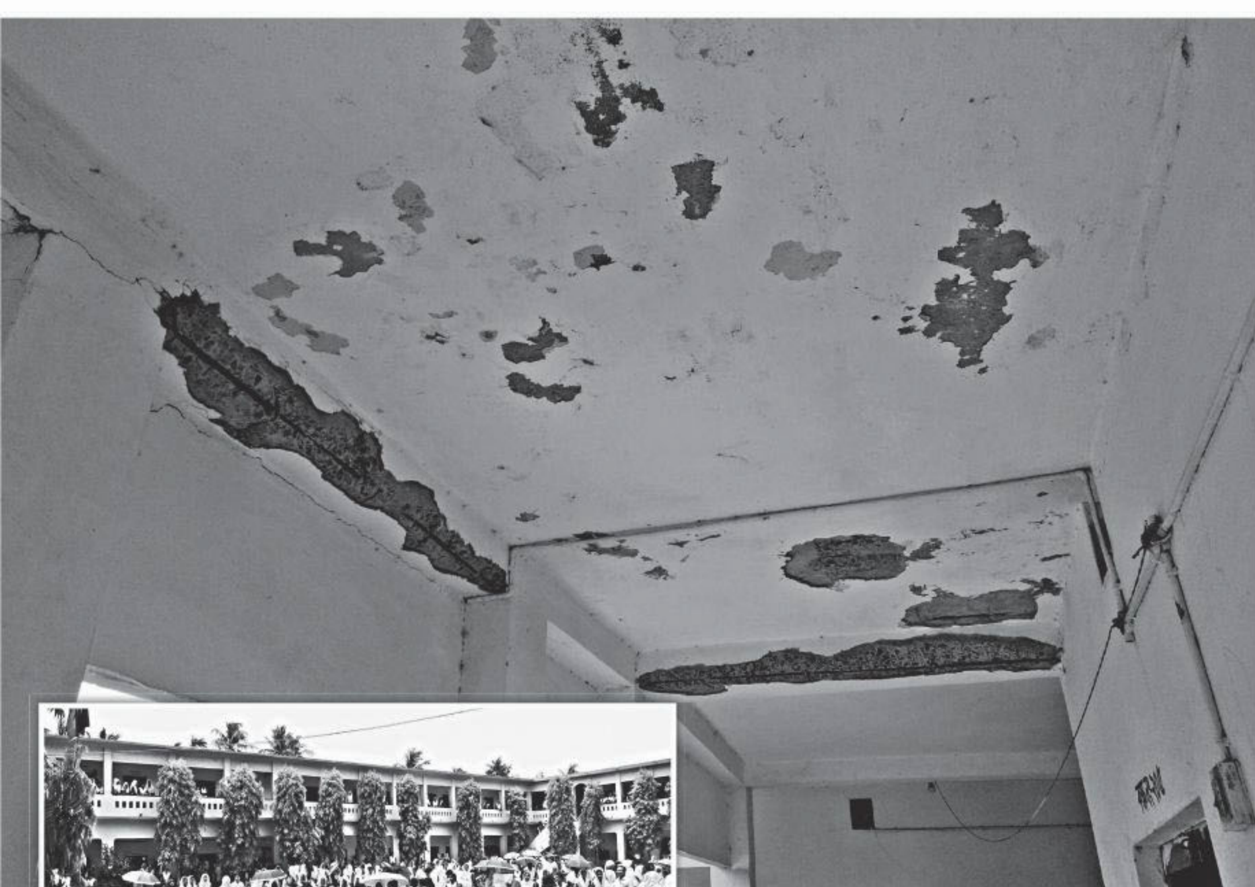
A portion of damaged ceiling in the hallway of the northern building of Kotchandpur Secondary Girls' School, inset, in Kotchandpur upazila town. The photo was taken recently.
