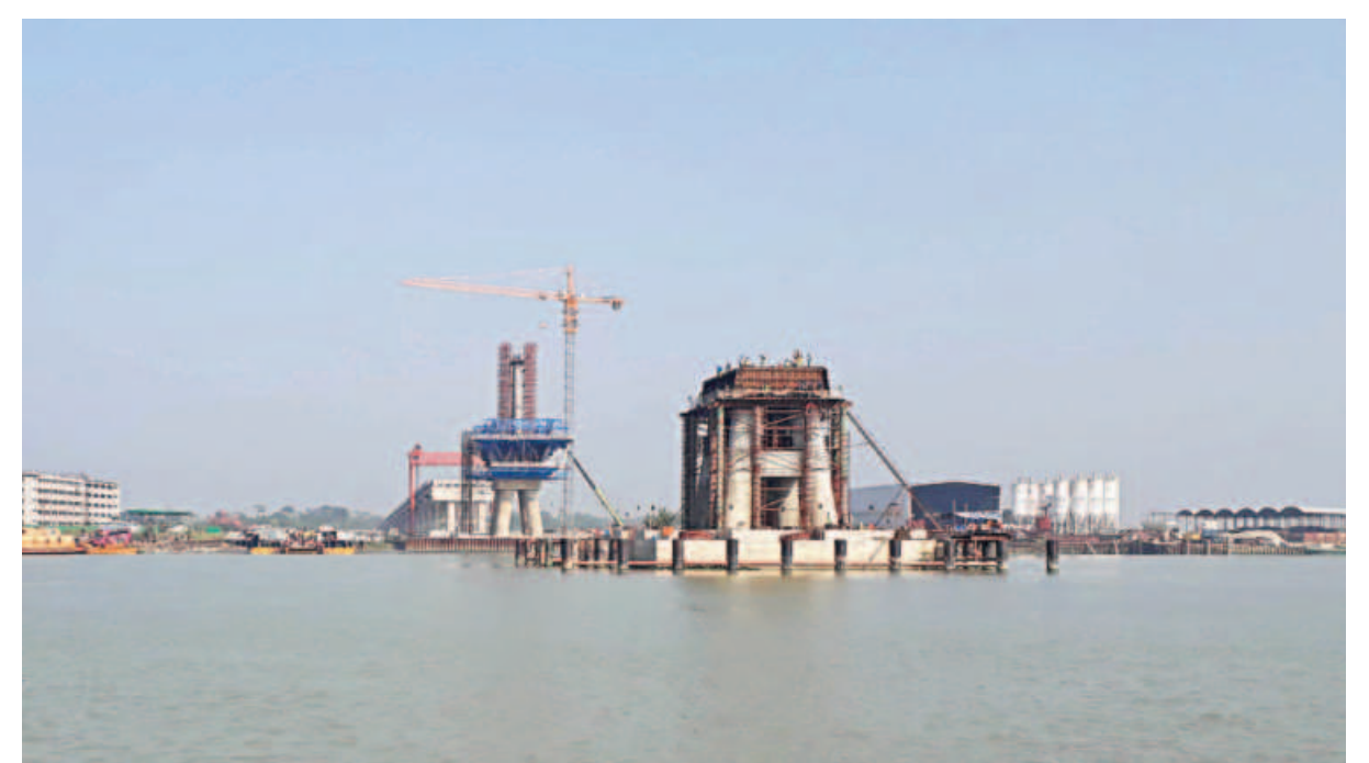
Construction work of Payra Bridge in Lebukhali area of Patuakhali is still incomplete although the scheduled completion date was April this year.
