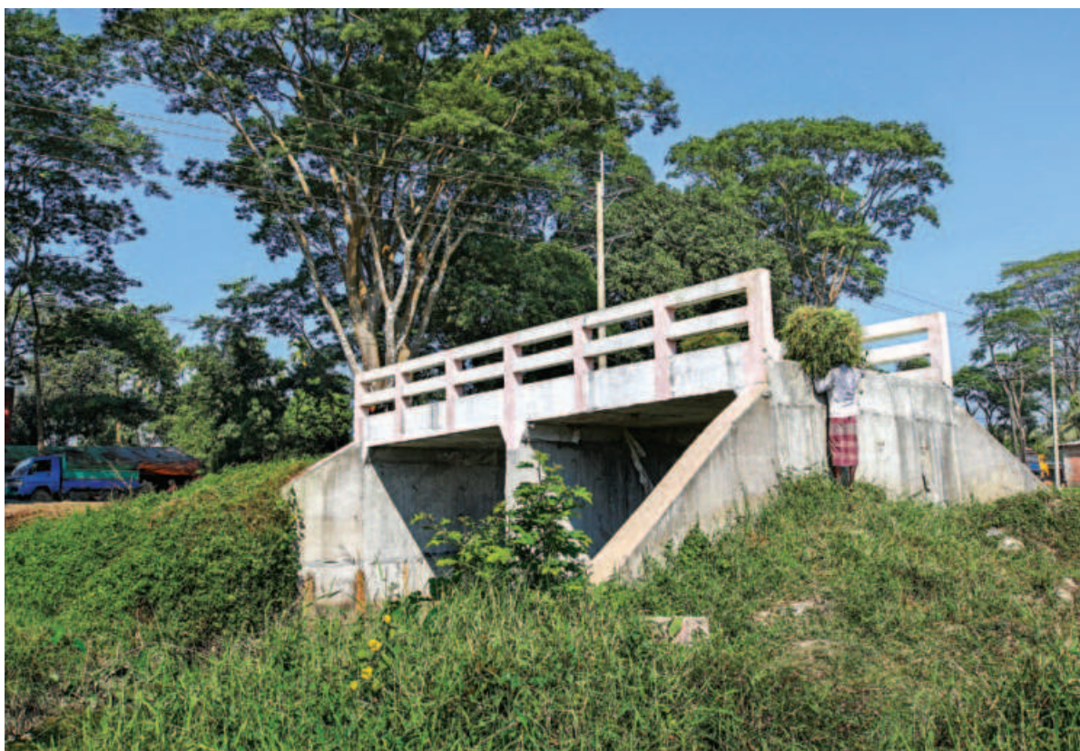
Going across this bridge in Phartali area of Chattogram's Raozan is not an easy feat. As no approach road has been built even an year after the bridge was constructed, villagers have to struggle a lot to use it. The photo was taken last week.
