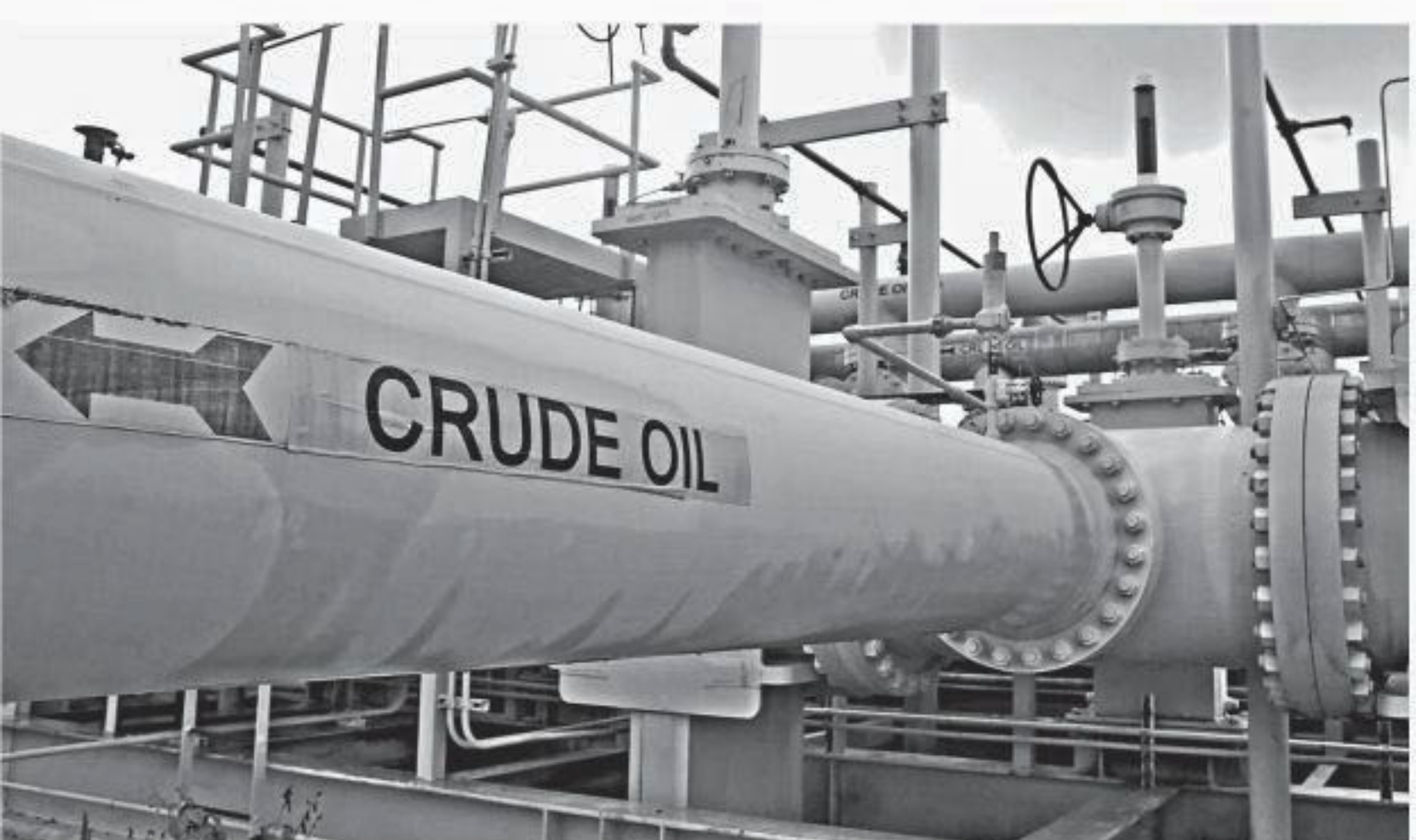
A maze of crude oil pipes and valves is pictured at the Strategic Petroleum Reserve in Freeport, Texas, US.
