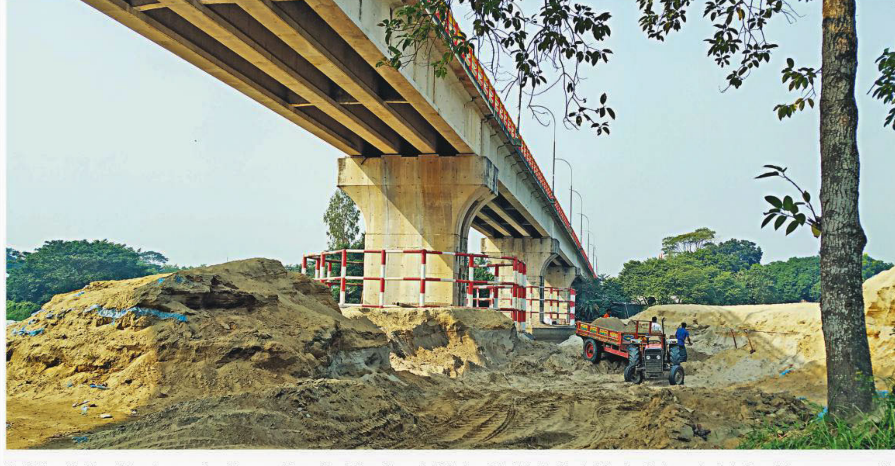
An influential local has been extracting sand from the Titas river, right below Sheikh Hasina bridge in Brahmanbaria's Banchharampur upazila. Several piers of the bridge have been made part of an enclosure for selling and stockpiling sand. The photo was taken recently. PHOTO: STAR
