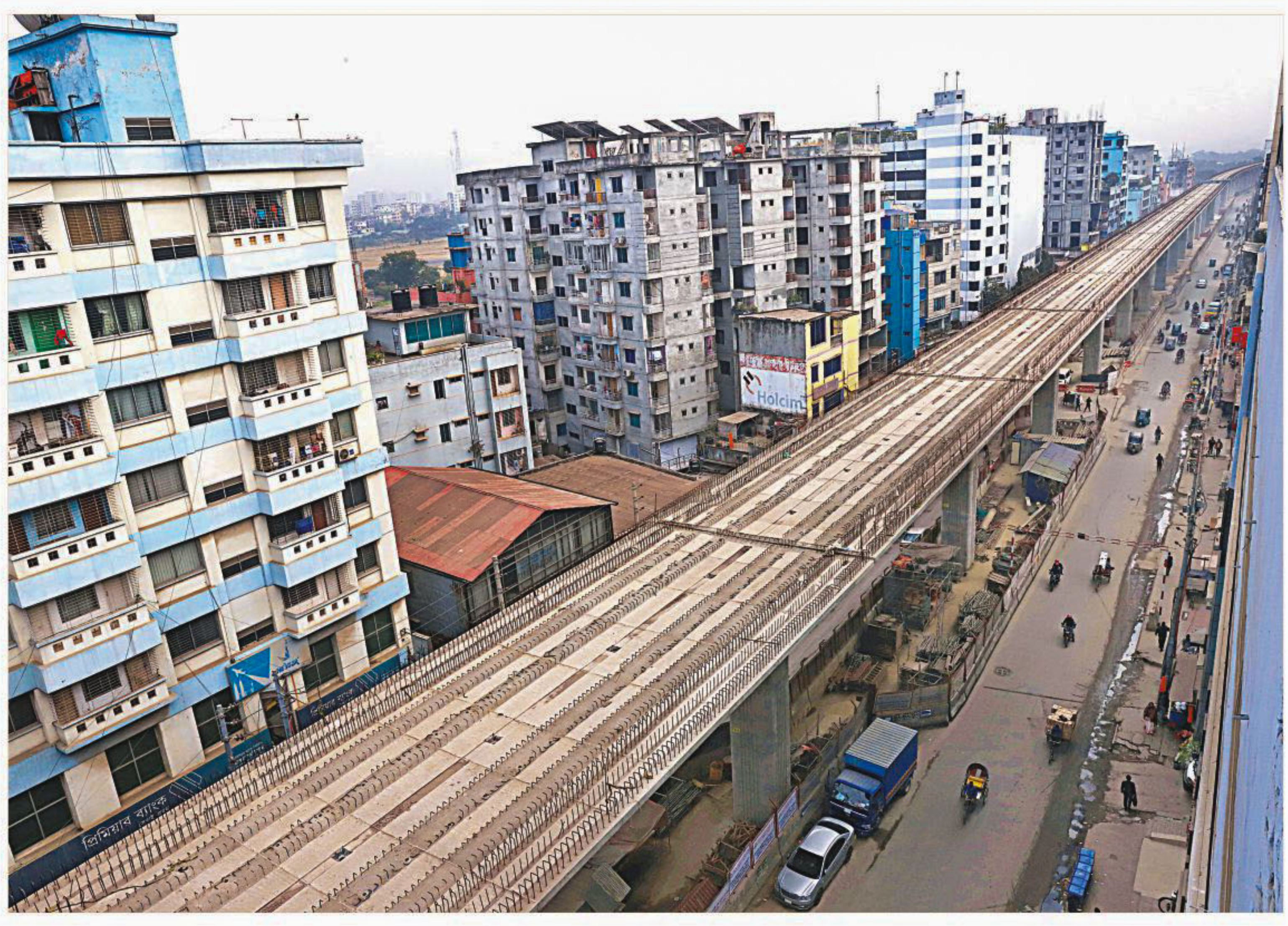
A portion of the metro rail's viaduct in Shewrapara in the capital. The project authorities are set to start installing rail lines on the elevated structure on January 1. The photo was taken yesterday. PHOTO: AMRAN HOSSAIN
