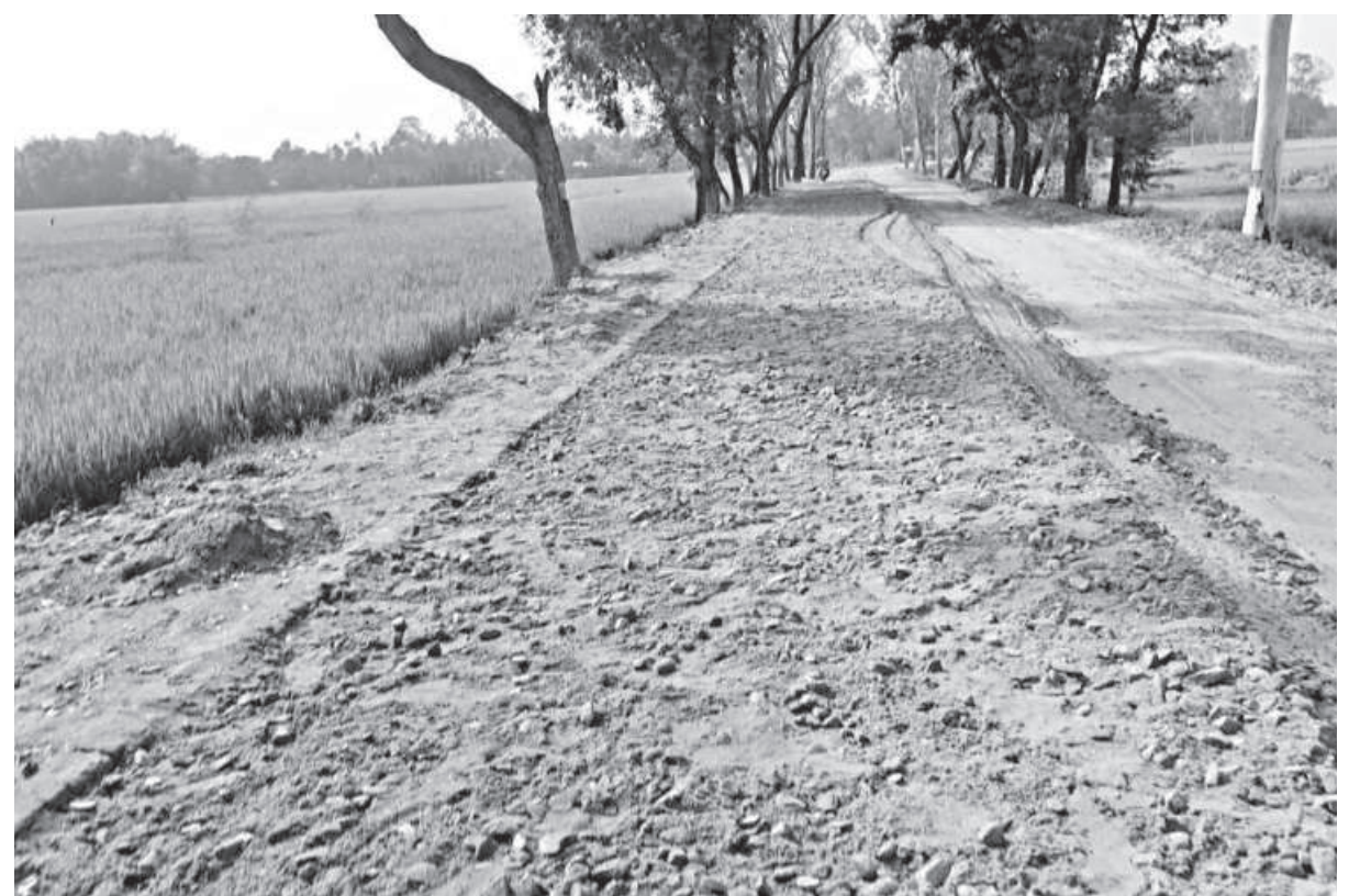
A section of Patgram-Dahagram road that is being reconstructed by Roads and Highways Department in Patgram upazila of Lalmonirhat. The photo was taken recently.
