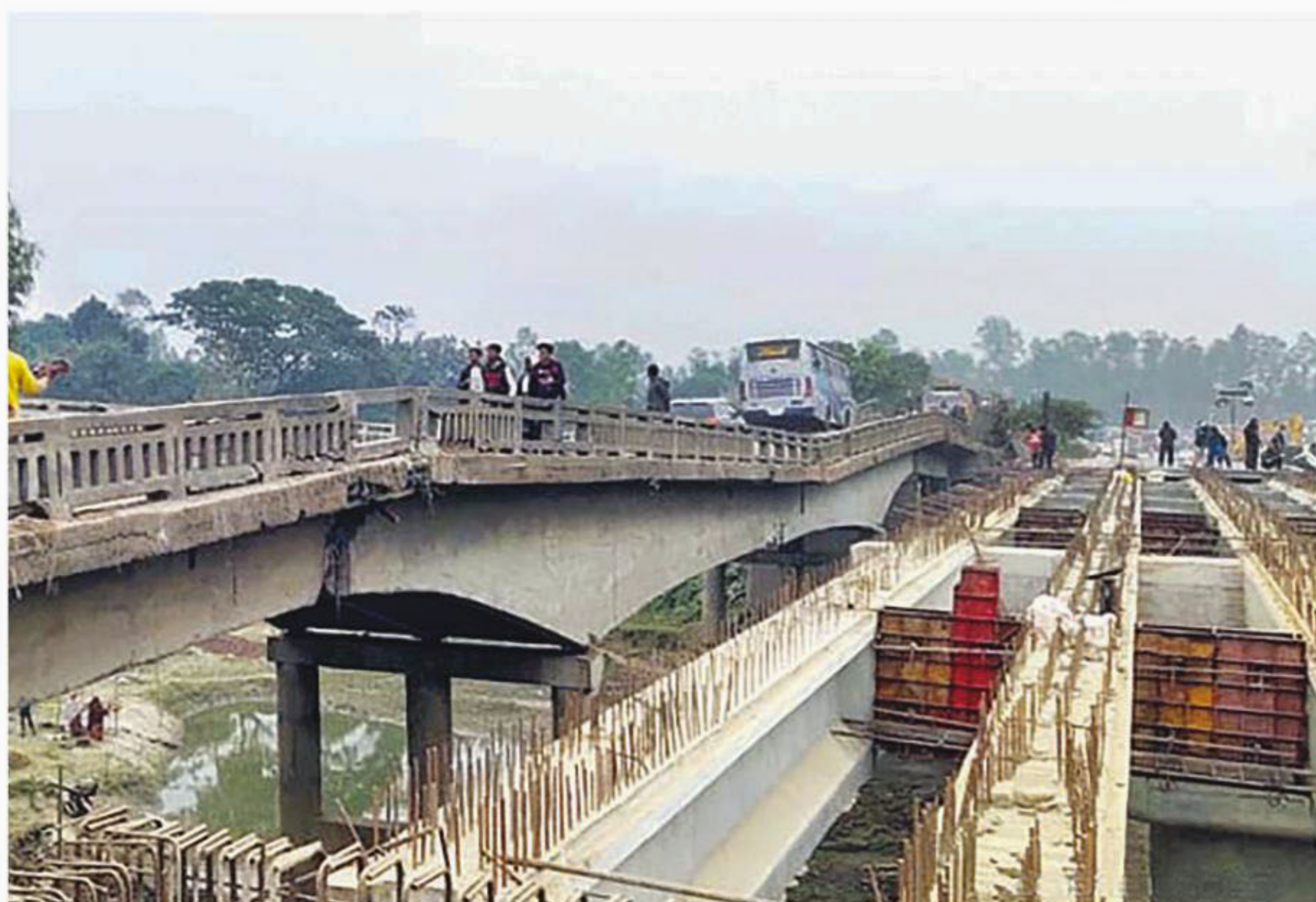
A part of this 80-metre bridge in Vuiagaati area of Sirajganj's Raiganj upazila subsided on Wednesday night, disrupting traffic movement on the Hatikumrul-Bogura highway. Construction of an alternative bridge, just beside the dilapidated one, has not ended in a year.
