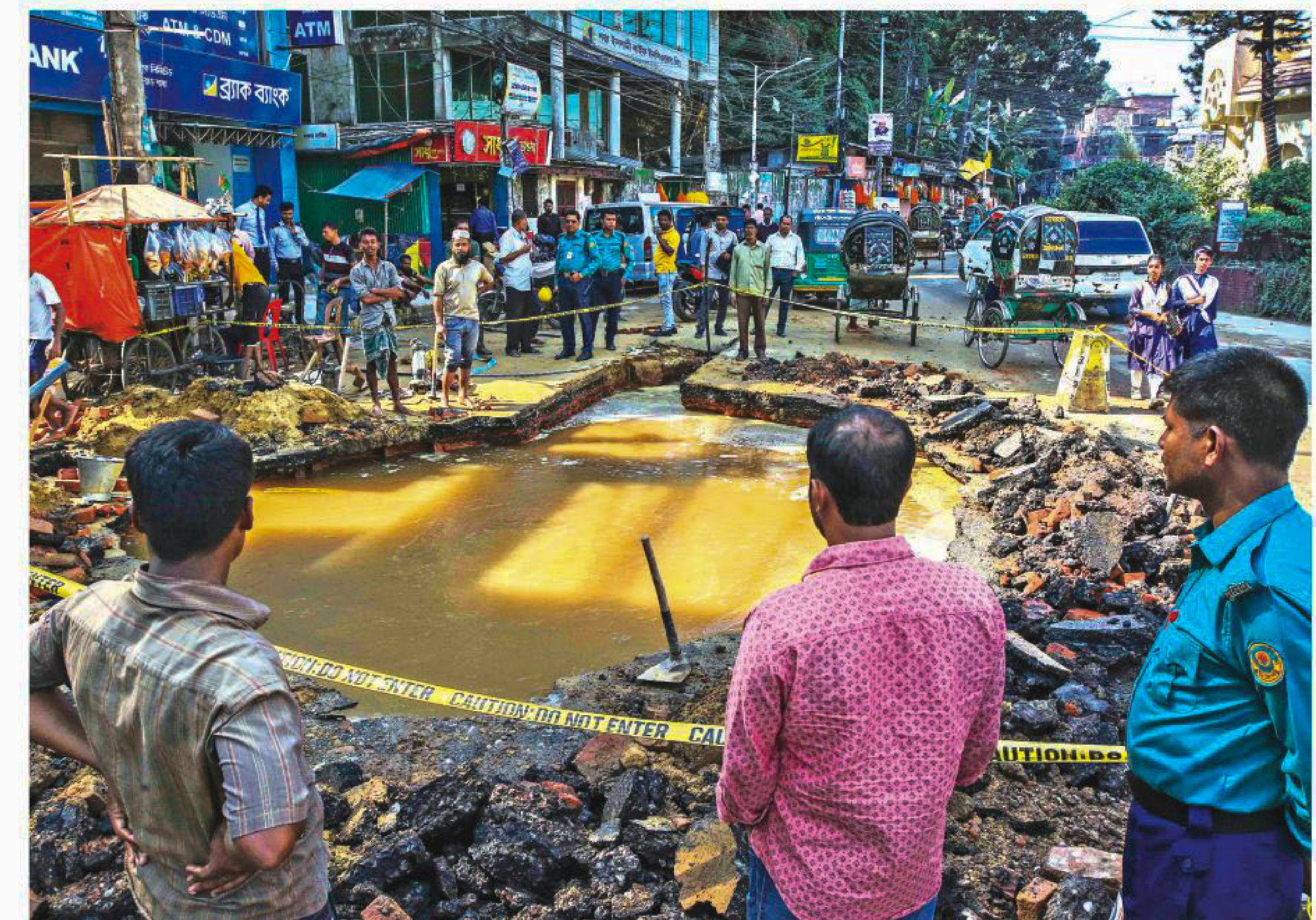
Locals surround a large puddle at Cheragi Pahar intersection in port city, cordoned off by Wasa after an underground pipe cracked around 8am yesterday and started leaking. According to locals, the incident took place while workers were installing cables there. When this photo was taken in the afternoon, Wasa workers were still fixing the leak.
