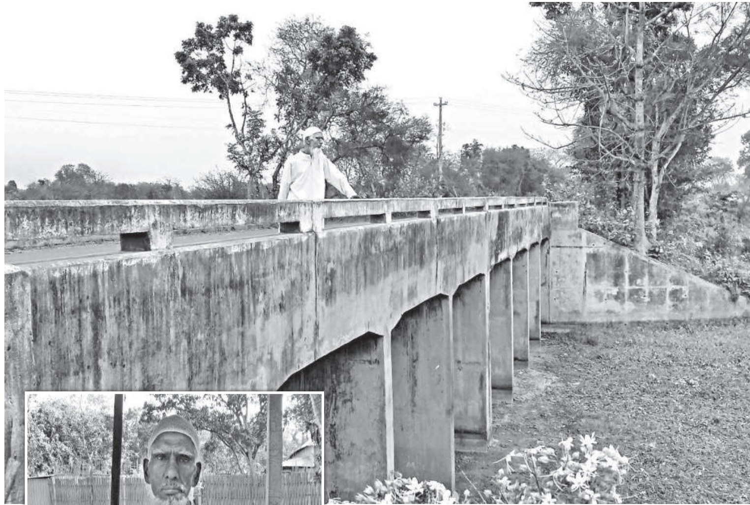
Sahab Uddin stands on the reconstructed Sholabaria Bridge in Pabna's Sujanagar upazila. He took part in the operation when the bridge was blown up on December 5 in 1971.
