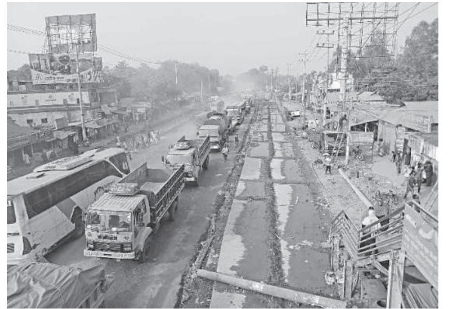
Hundreds of vehicles on Dhaka-Tangail highway remain stuck in a long tailback for the last two days due to road-widening work at Elenga.
