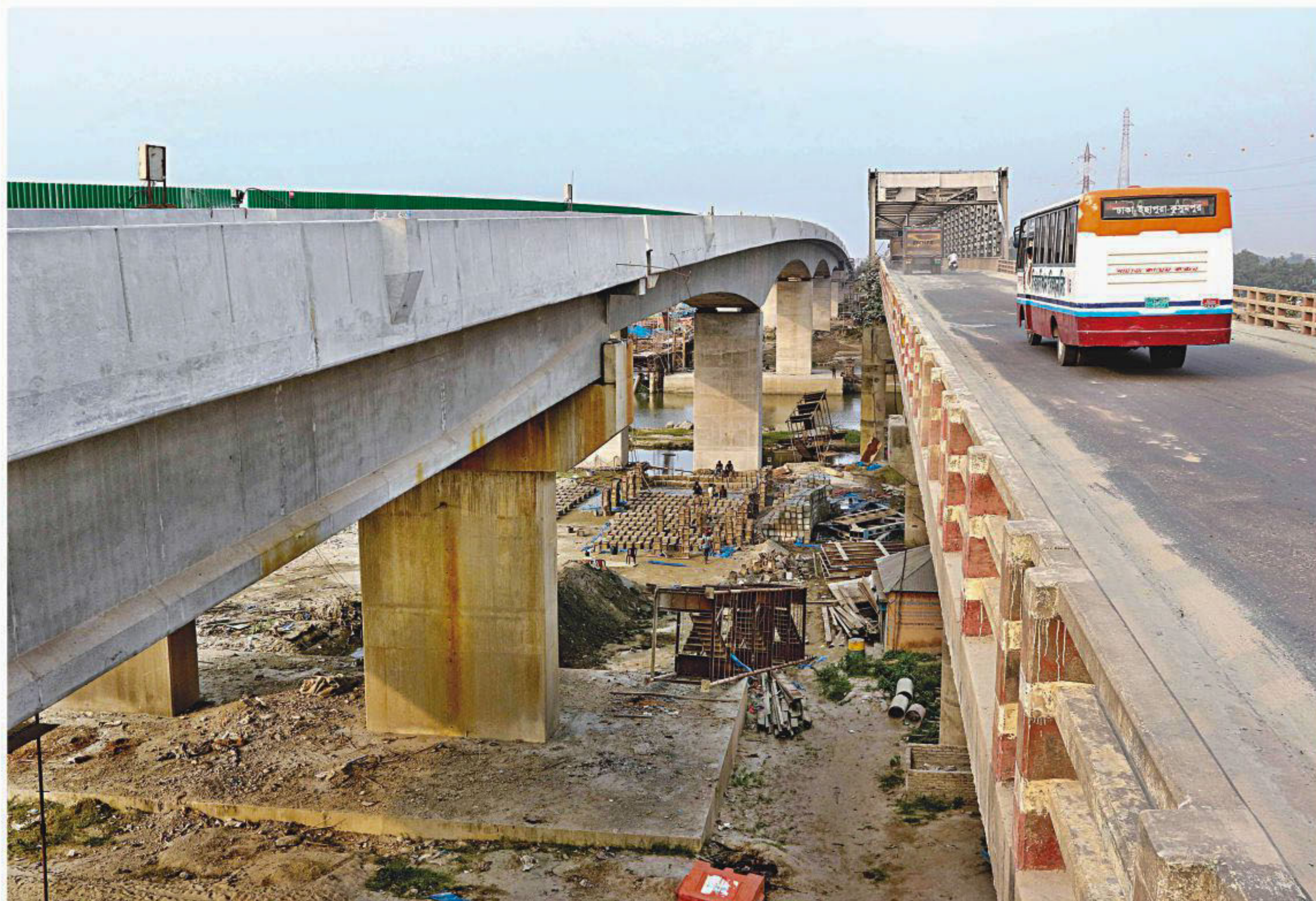
A new bridge is being built alongside the existing Dhaleshwari bridge on Dhaka-Mawa highway in Munshiganj. The new bridge, likely to be opened in June next year, will facilitate smooth flow of traffic on the highway after the inauguration of Padma bridge. The photo was taken recently.
