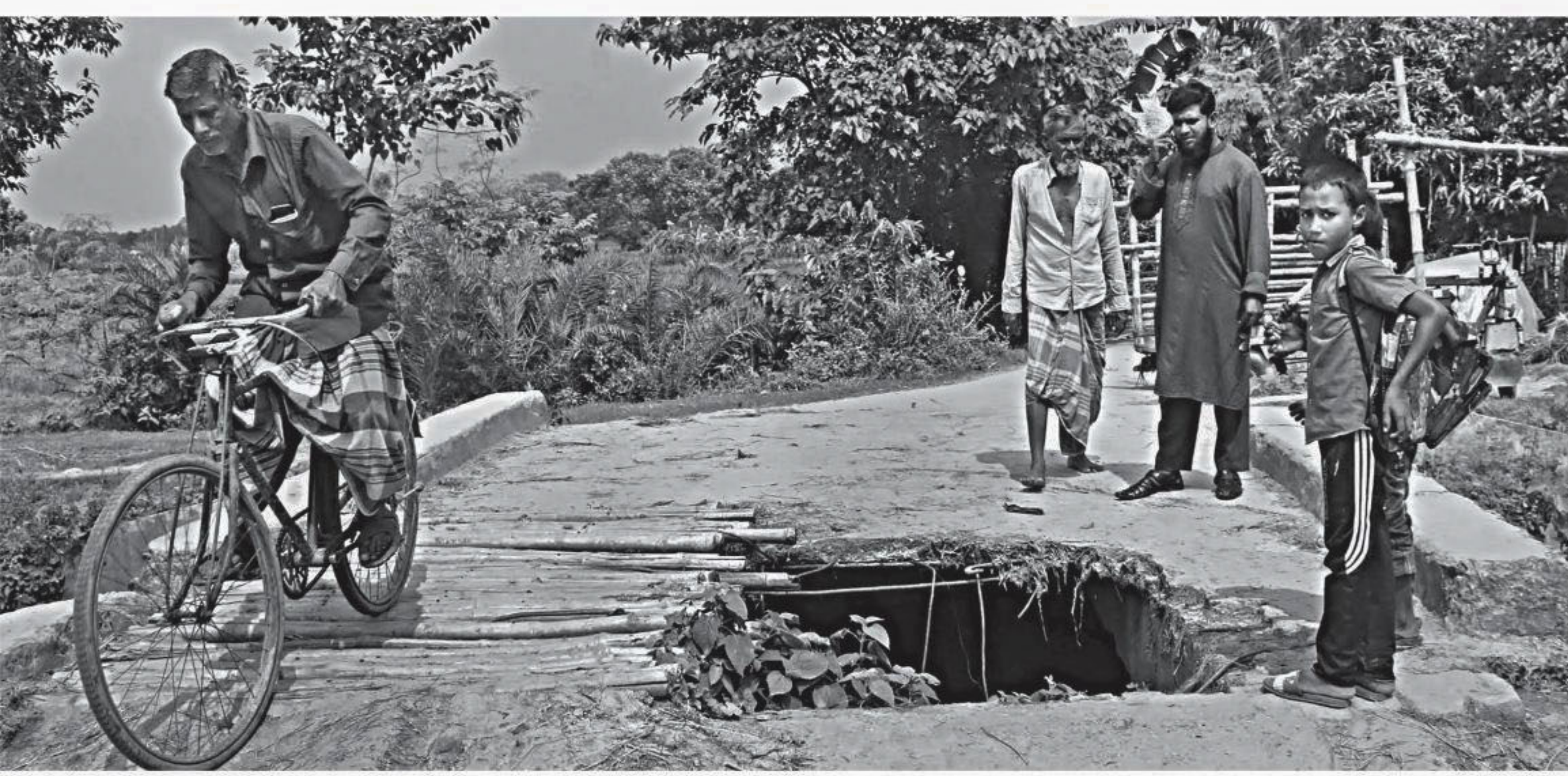
A man pedals his bicycle over the bamboo platform that the villagers put on a broken section of the bridge on the road between Harinakundo upazila town and Daulatpur bazar in the same upazila. The photo was taken recently.
