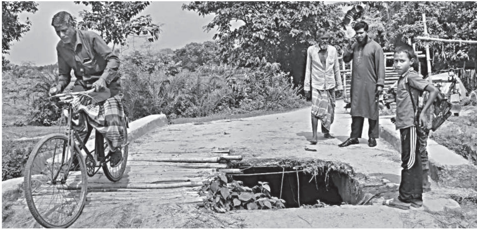
A man pedals his bicycle over the bamboo platform that the villagers put on a broken section of the bridge on the road between Harinakundo upazila town and Daulatpur bazar in the same upazila. The photo was taken recently.
