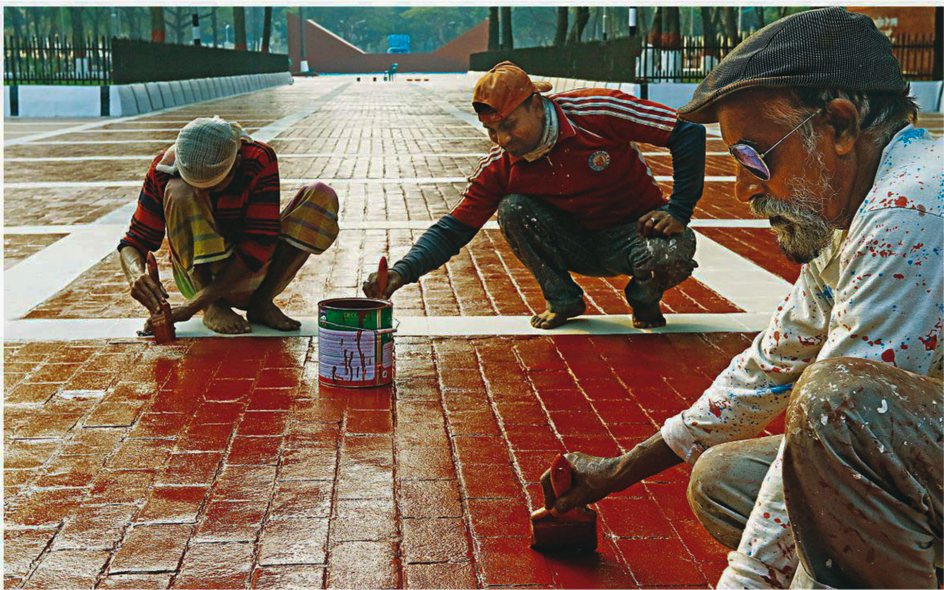
Dhaka North City Corporation has been sprucing up the memorial for martyred intellectuals in Mirpur ahead of Martyred Intellectuals' Day on December 14. This photo of workers painting the surface as part of the initiative was taken yesterday.
