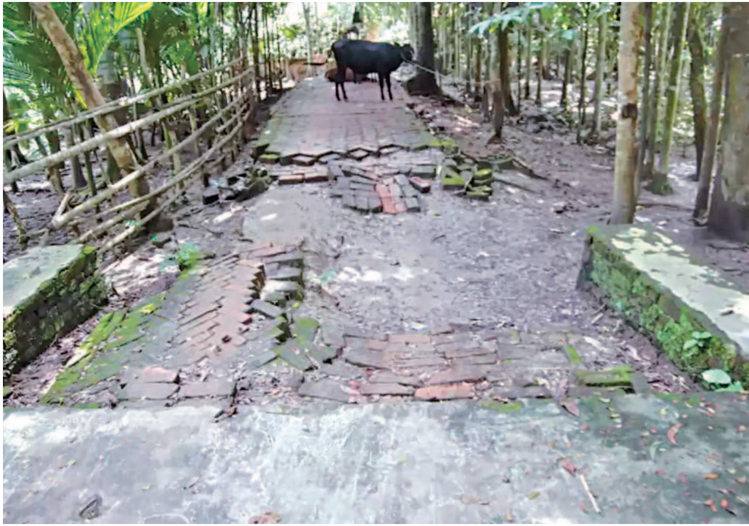
A village road in Jhalakathi's Rajapur upazila lies in awful state for years, causing immense sufferings to commuters. PHOTO: STAR
