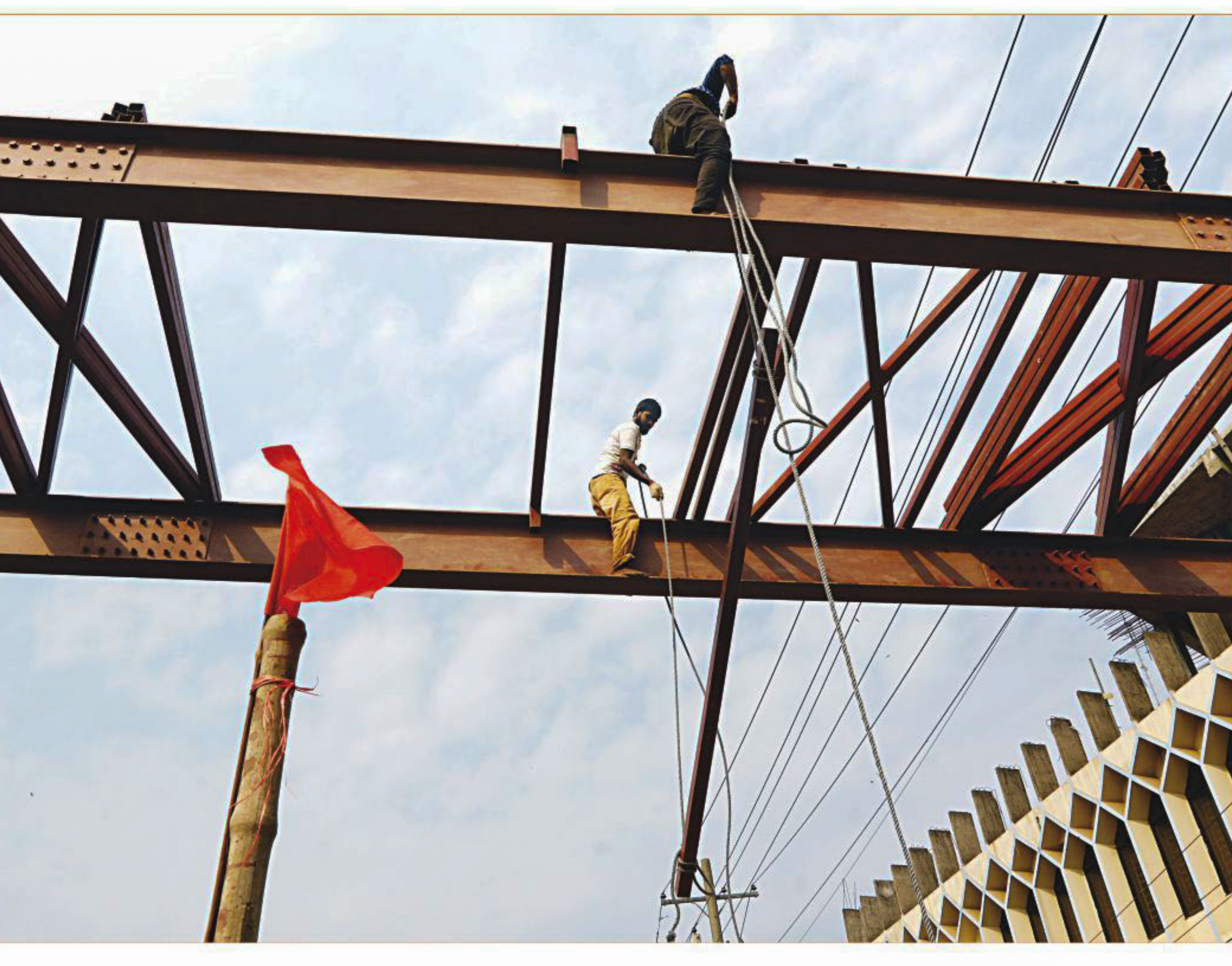
A red flag flutters in the wind, while two labourers, without wearing any safety gear, work on top of an under-construction footbridge in Aminbazar on the Dhaka-Aricha highway yesterday. The flag is supposed to warn pedestrians of the ongoing construction overhead, but little regard for safety is shown for the workers engaged in the construction itself.
