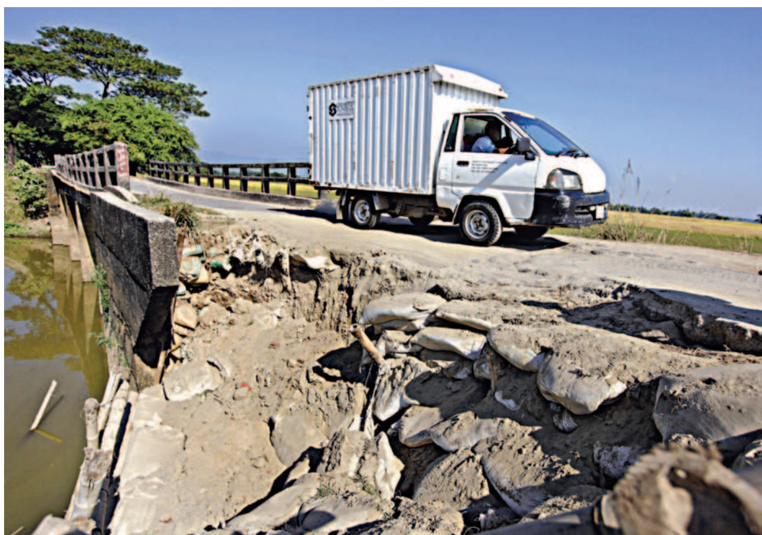
A van crosses a badly damaged bridge in Paschim Jaflong Chotkhel area in Sylhet's Gowainghat upazila yesterday. Locals said part of the bridge's approach road caved in six months ago, after which the LGRD did some makeshift repairs using sandbags and bamboos. Those too were flooded away by recent rains.
