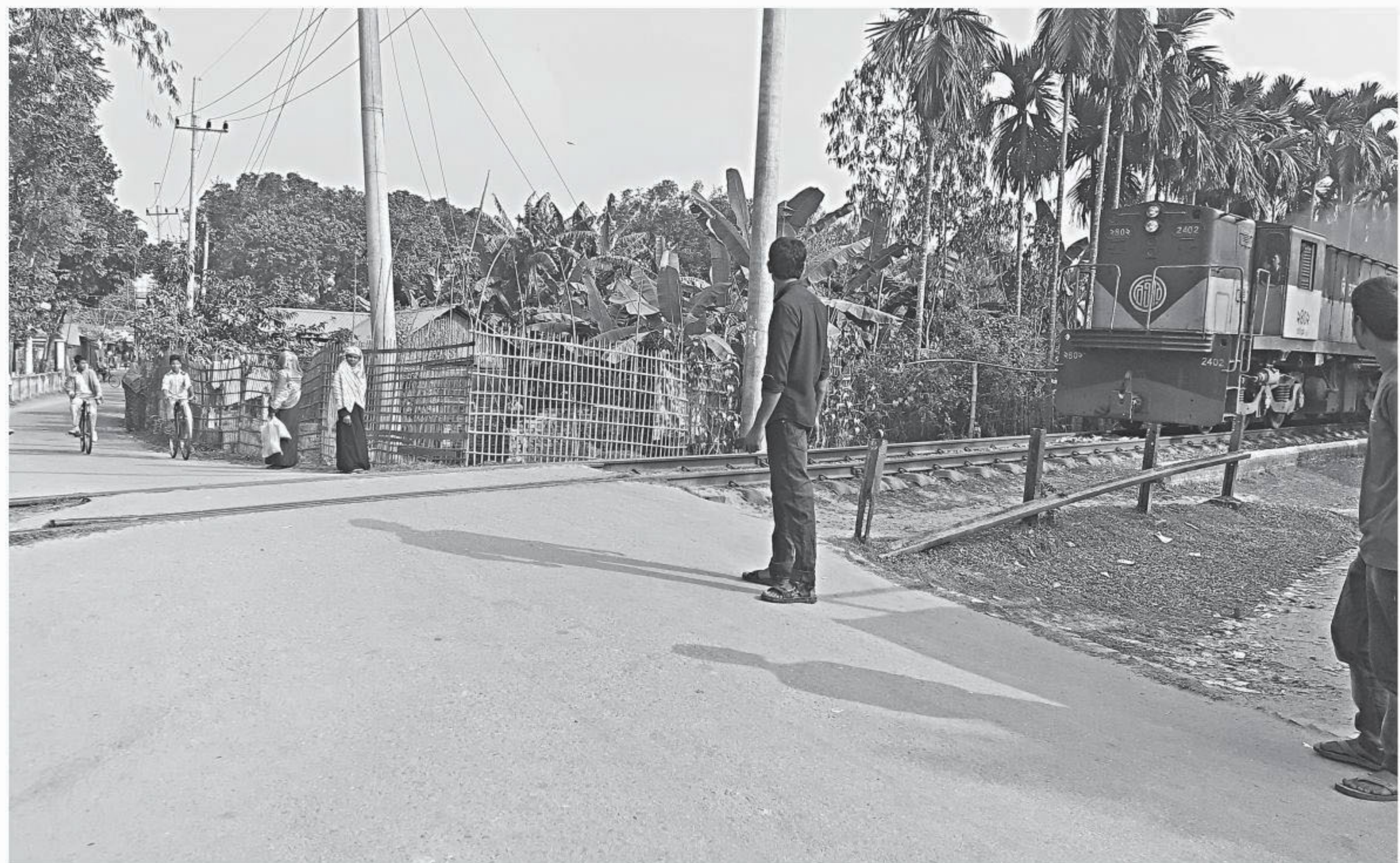
A level crossing on BDR road in Lalmonirhat town has remained without gate and gateman, posing risk of fatal accidents. The photo was taken on Monday.
