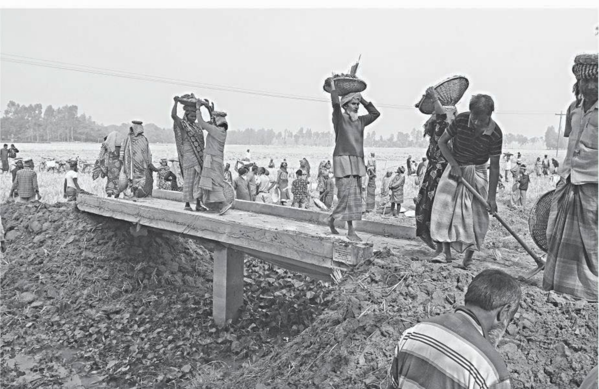
Labourers, enlisted under the government's 40-day job scheme, are engaged in constructing approach roads on either sides of a bridge over a canal, built by Panchara Union Parishad in Naogaon's Patnitola upazila. The bridge has been lying useless for months for want of approach roads.
