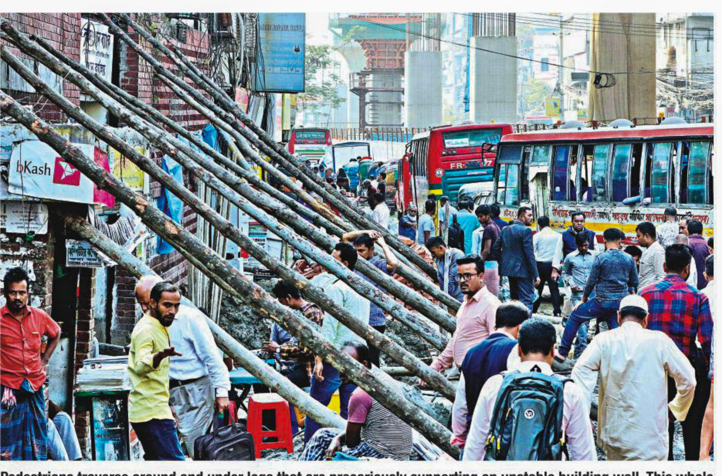
Pedestrians traverse around and under logs that are precariously supporting an unstable building wall. This whole situation is a result of authorities digging up the road for sewage line work. This photo was taken on Tuesday near Dainik Bangla intersection. PHOTO: ANISUR RAHMAN
