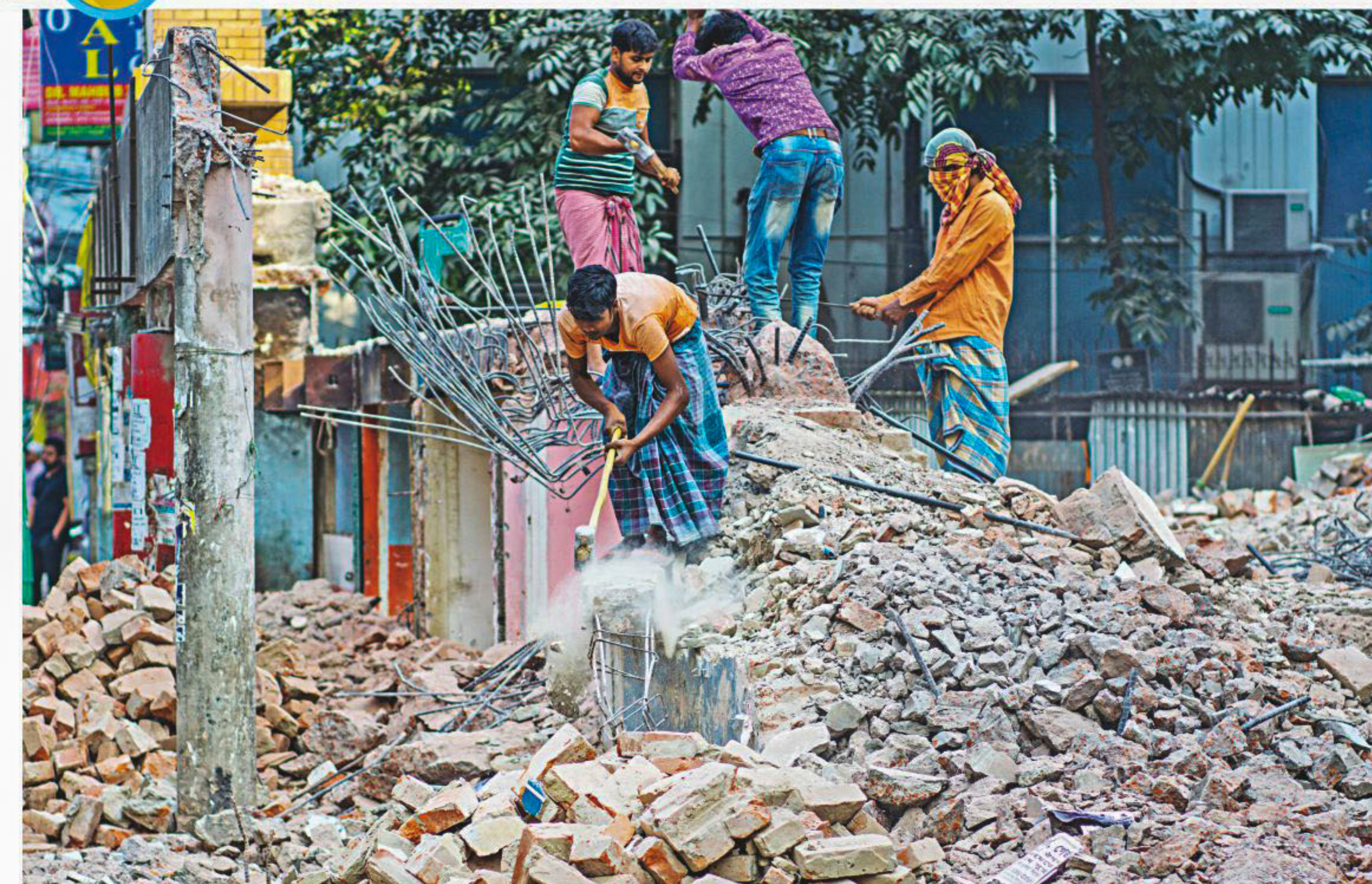
Demolition work of a building goes on in the capital's Kalabagan without any measures to contain the dust and debris, as Dhaka continues to grapple with severe air pollution this dry season. Despite directives from the High Court to ensure construction sites are kept covered and water is sprinkled at places where a lot of dust may be produced, such scenes are common across the city.
