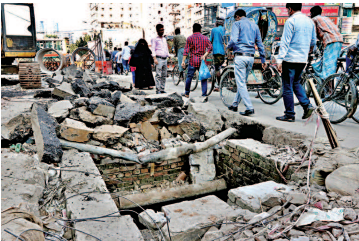
Part of a road dug up for work on storm drainage in the capital's Dainik Banglar intersection poses danger to vehicles and pedestrians. Locals said the road has been in this state for at least a couple of months. The photo was taken on Wednesday.
