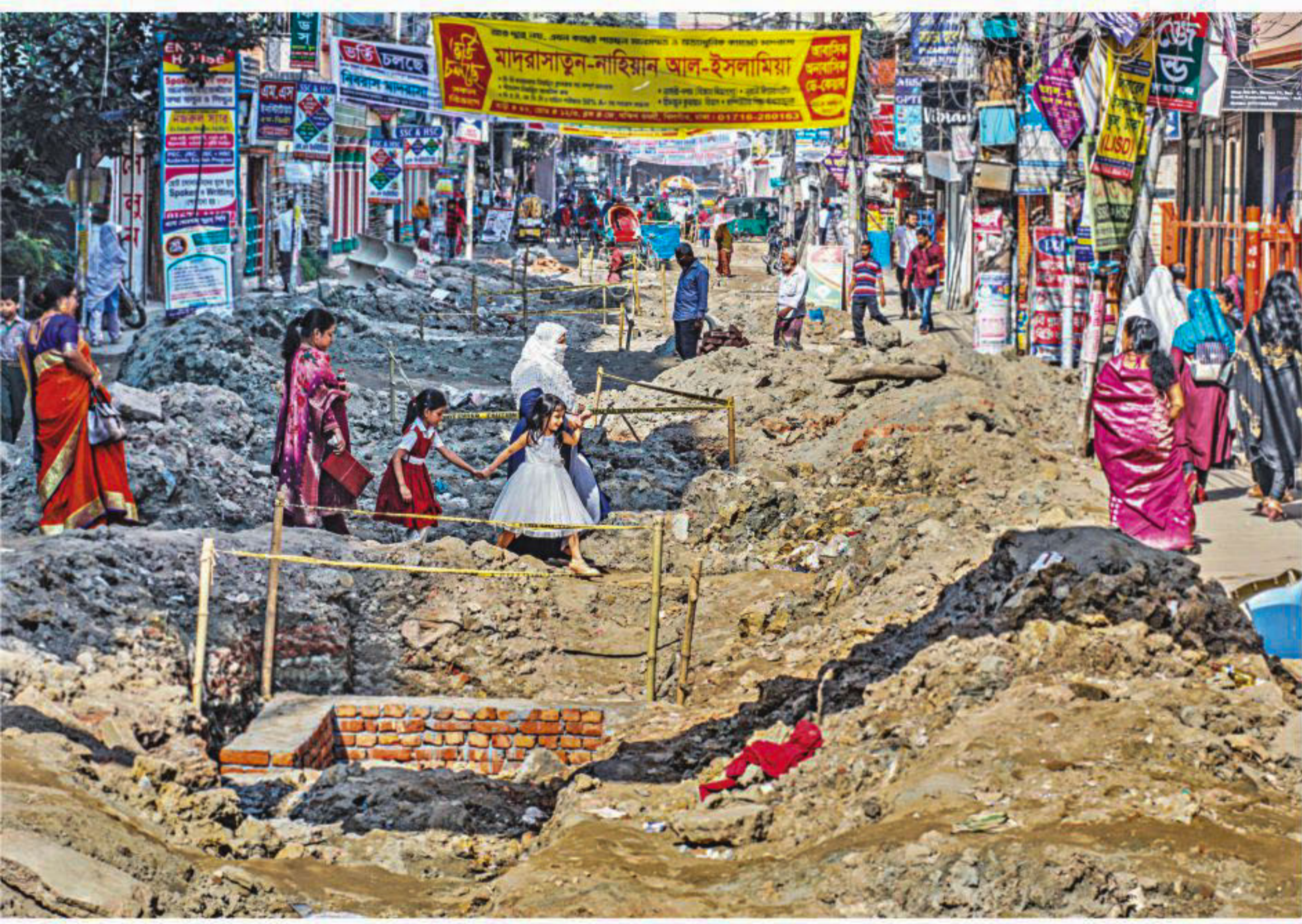
The city corporations are installing sewage lines in South Banasree road at a snail's pace. Locals have been putting up with the dug-up road for almost a year now. The photo was taken yesterday.
