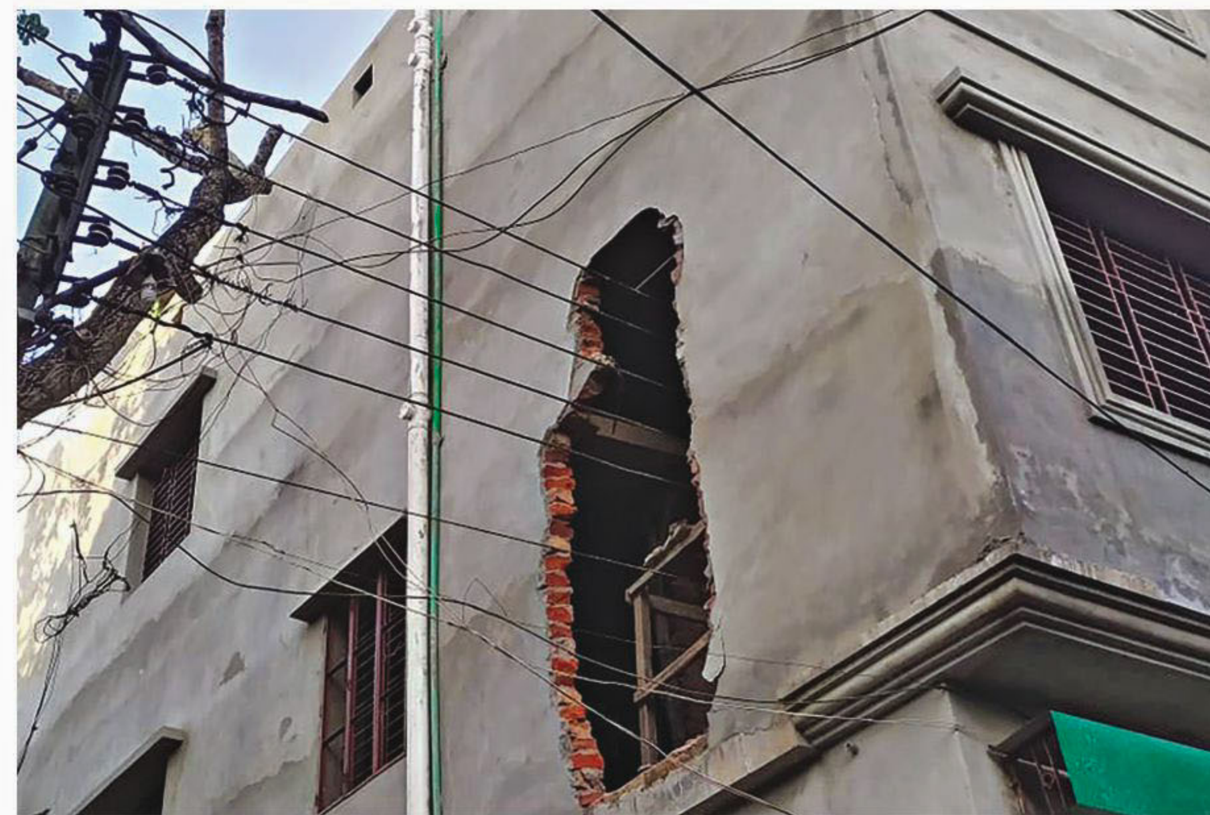
FLIRTING WITH DANGER ... High-voltage electric cables go through an under-construction building on BT Road in Chandpur town. The authorities say they will soon take action against the owner for constructing the building illegally and ignoring the risks. The photo was taken on Wednesday afternoon.
