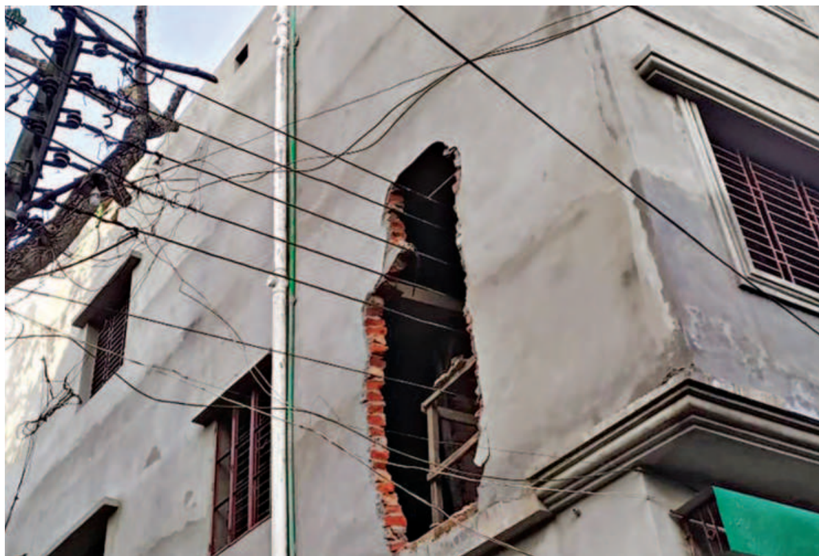
FLIRTING WITH DANGER ... High-voltage electric cables go through an under-construction building on BT Road in Chandpur town. The authorities say they will soon take action against the owner for constructing the building illegally and ignoring the risks. The photo was taken on Wednesday afternoon.
