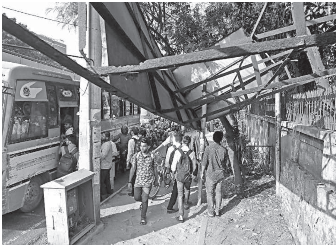
Rusted iron bars of what was once a passenger shed at a bus stop now hangs precariously over pedestrians, threatening to collapse at any time. The photo was taken yesterday from the capital's Tejgaon Satrasta.
